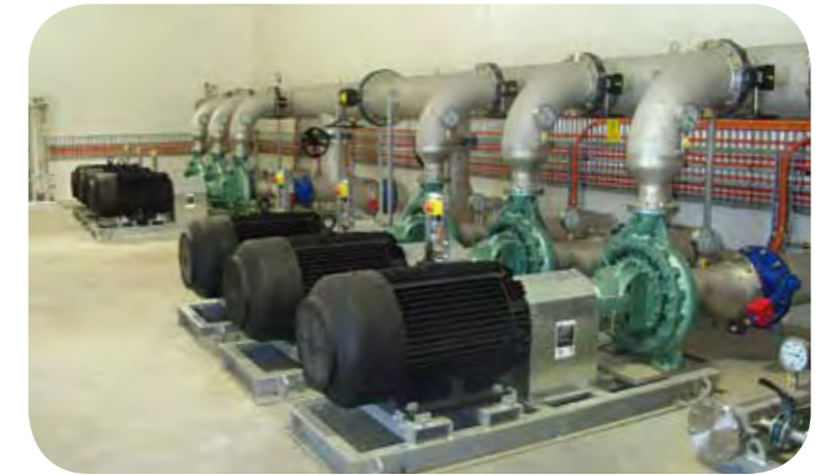
Longerenong pump station
