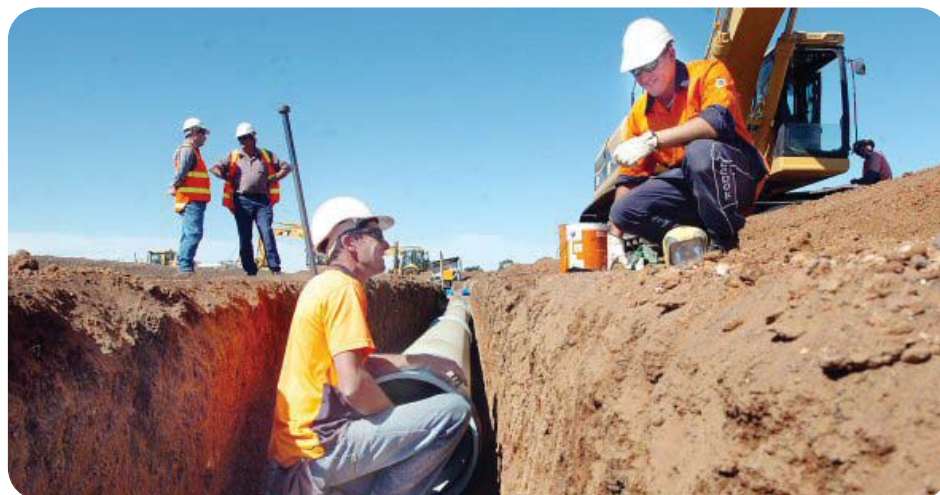
Pipe laying contractors on-site near Dooen Photo courtesy of Michael Rudolph, Wimmera Mail-Times
