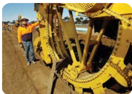
A Cleveland trencher lays 450 mm pipe near Dooen Photo courtesy of Michael Rudolph, Wimmera Mail-Times
